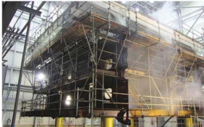
FPSO P66 being assembled (top), block being UHP waterjetted inside blasting chamber (above) and surface-tolerant coating being applied (right).
