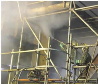
Second system coat being applied (top left), electrically operated UHP waterjetting machines working at 40,000 psi (top right) and worker waterjet cleaning to SSPC-SP WJ-2/ NACE WJ-2 standard (above).
